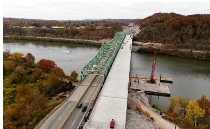
Figure 18: The second project widened the bridge pictured here, with contra flow while constructing.
