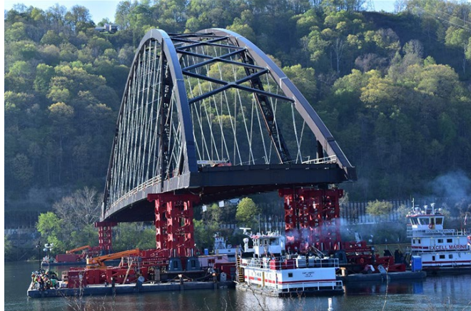
Figure 17: One of the West Virginia bridges recently constructed, connecting Ohio and West Virginia. It weighs 4800 tons without concrete and rebar. To place the structure, it was floated down the river and erected in place.
